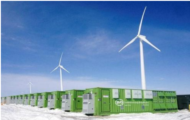
Energy storage system
